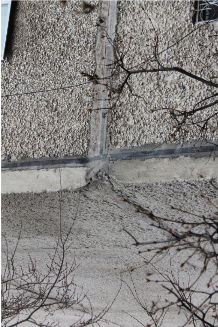
Figure 2.8: Cracking of the joint reported in building 4/1, documented during the second inspection. The shape of the crack led us to believe that this could become a local point of failure in case of large ground motion excitation.
