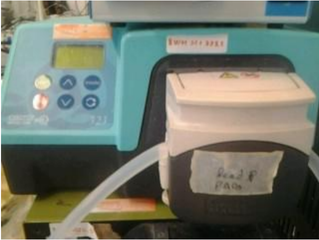
Figure 25. Pump for the phosphorus feeding to Acc. reactor
