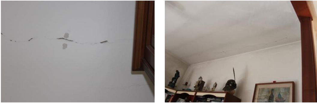
Figure 4.2 Cracks on the plasterwork
