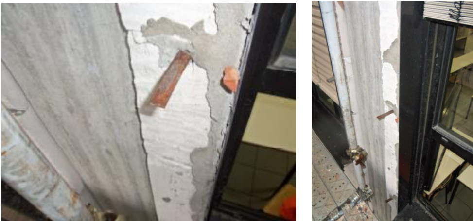
Figure 4.21 Connection element near the windows and in the jambs between the windows
