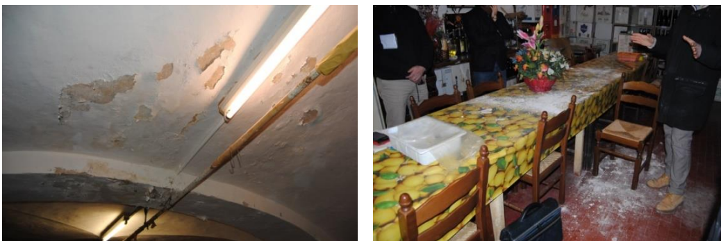
Figure 4.12 Deterioration of the surface due to infiltration of water
