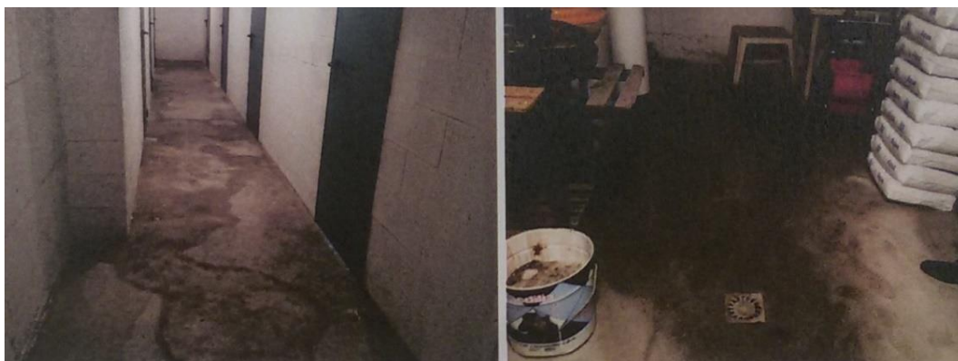
Figure 4.14 Stain on the flooring due to water stagnation
