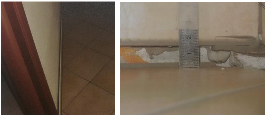
Figure 4.19 Detachment of the base board
