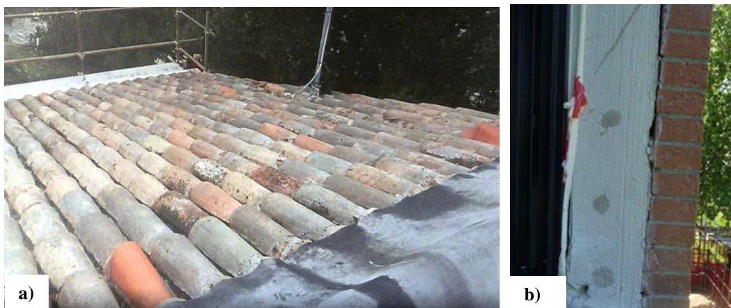
Figure 6.76 Examples of damage/deterioration: a) Shingles deterioration; b) Covering detachment
