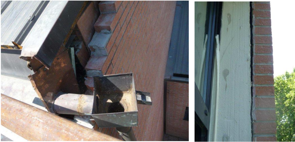
Figure 4.20 Collapse of the top part of the front and detachment of the wall covering
