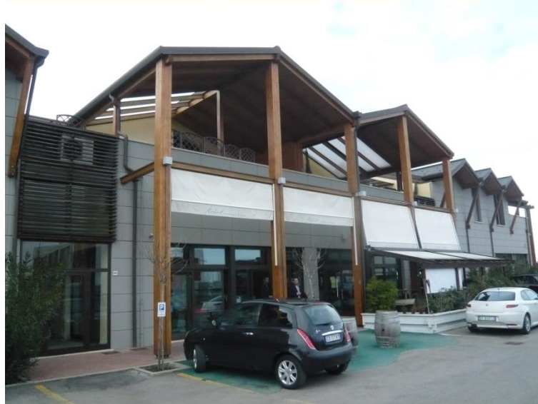
Figure 4.26: Degradation of a wood roofing
