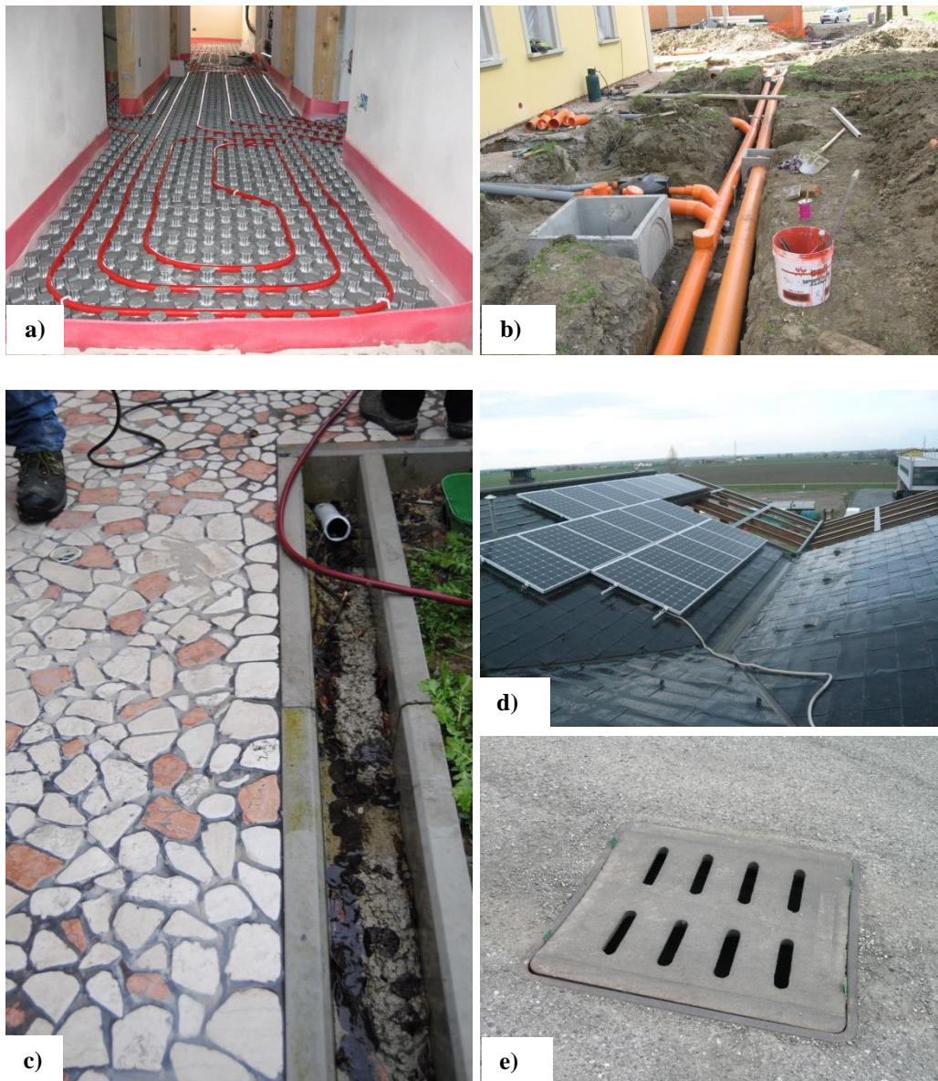
Figure 6.69 Examples of plants: a) Ground heating system; Wayer distribution system; c) Rain water removal system; d) Solar panels; e) gallipot
