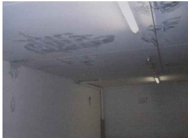
Figure 4.5 Water infiltration evidence on a ceiling
