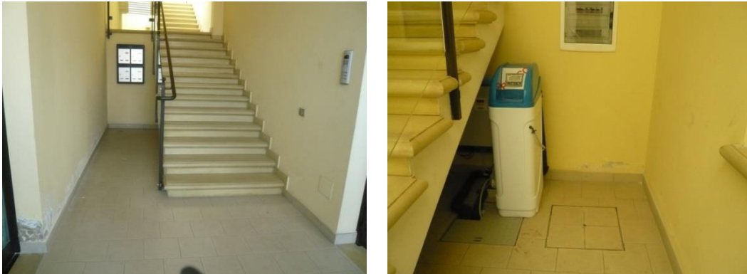
Figure 4.4 Evidence of dampness on the walls
