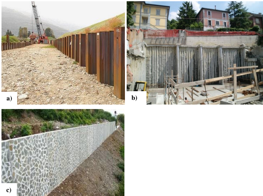
Figure 6.61 Examples of retaining structures: a) Sheet piles; b) Diaphragm wall; c) Retaining wall
