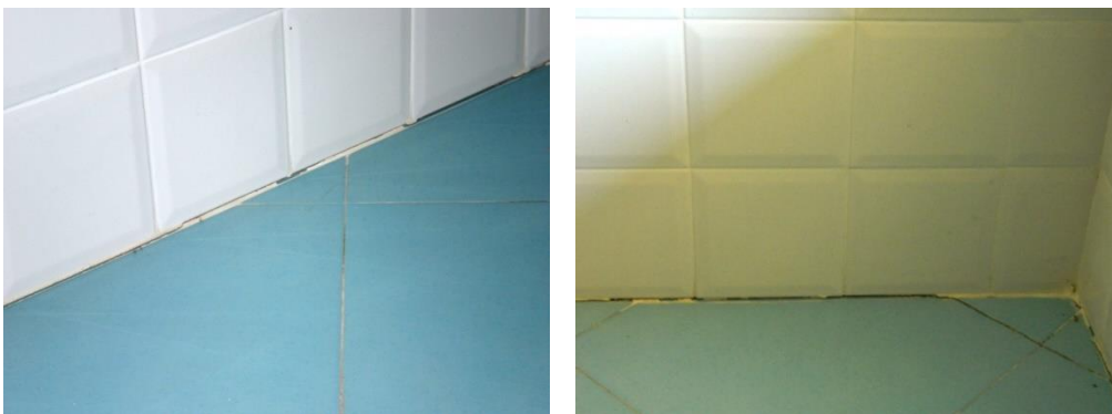
Figure 4.9 Detachment between the flooring and sealing of the wall
