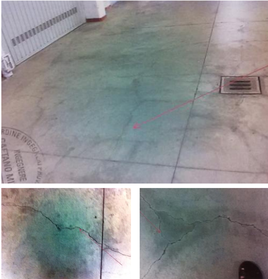
Figure 4.32 N° R.G. 2188/2012 Crack on the concrete flooring of a garage
