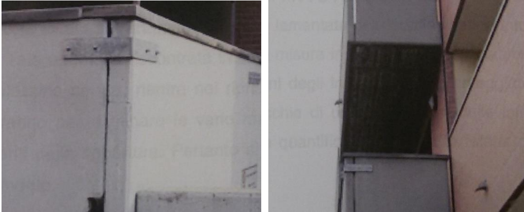
Figure 4.18 Instability of the railing of the building
