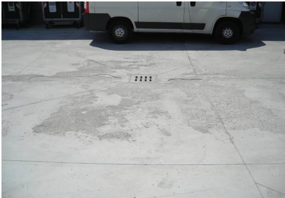
Figure 4.27 Crumbling of and industrial flooring
