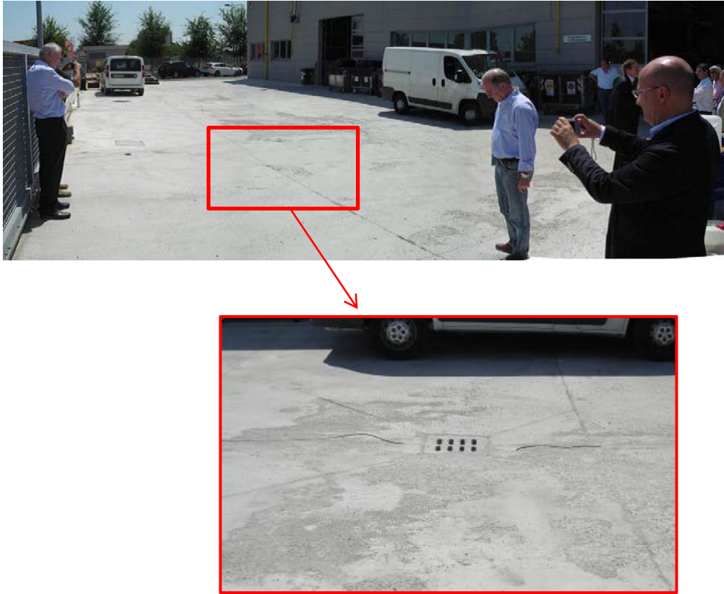
Figure 4.34 Crumbling of an external industrial flooring
