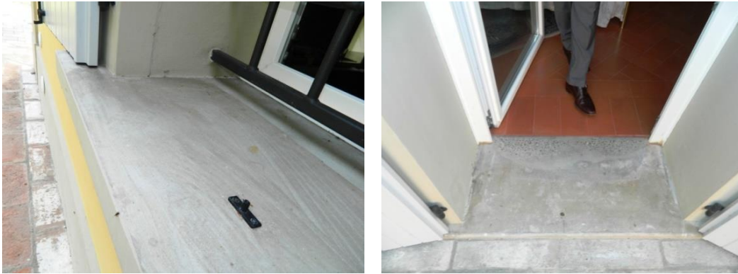
Figure 4.6 Cement stains on the windows sills and thresholds
