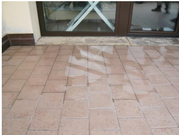
Figure 4.15 Water stagnation on a balcony
