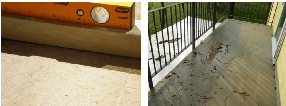
Figure 4.16 Water stagnation due to inadequate slope
