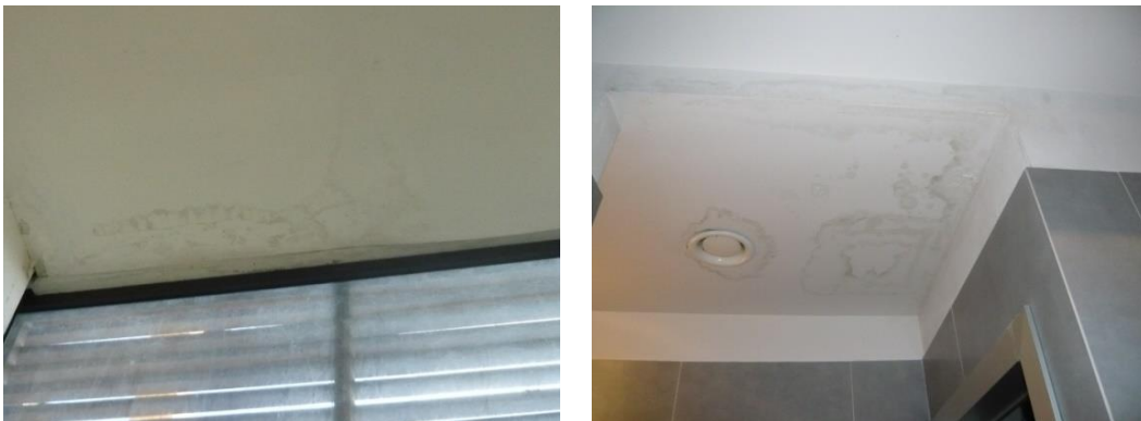
Figure 4.3 Dampness patches on the intrados of the slab
