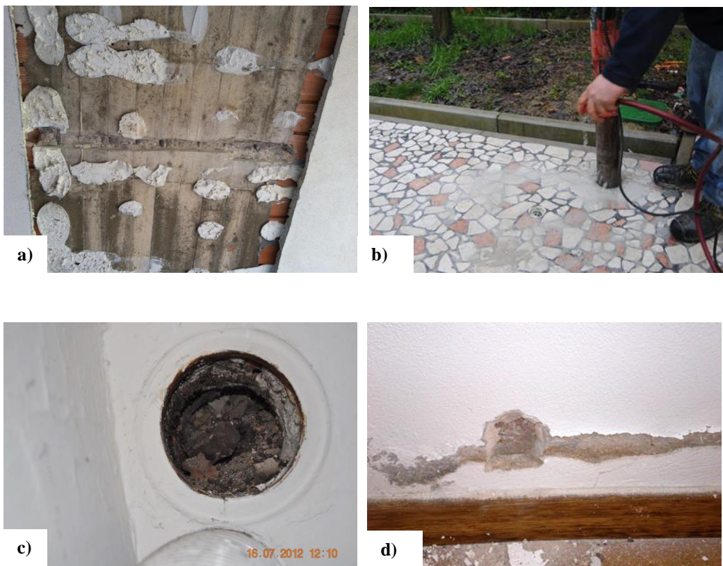
Figure 6.83 Examples of in situ test: a) Excavation of a beam b) Sampling of an external flooring; c) inspection hole for an exhaust pipe; d) Survey on a wall
