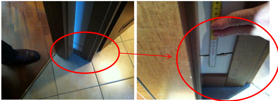
Figure 4.10 Large crack on the wall
