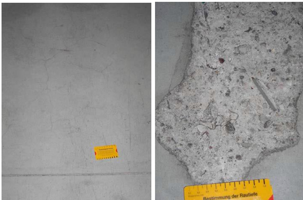
Figure 4.35 N° R.G. 6314 Delamination of an internal concrete flooring
