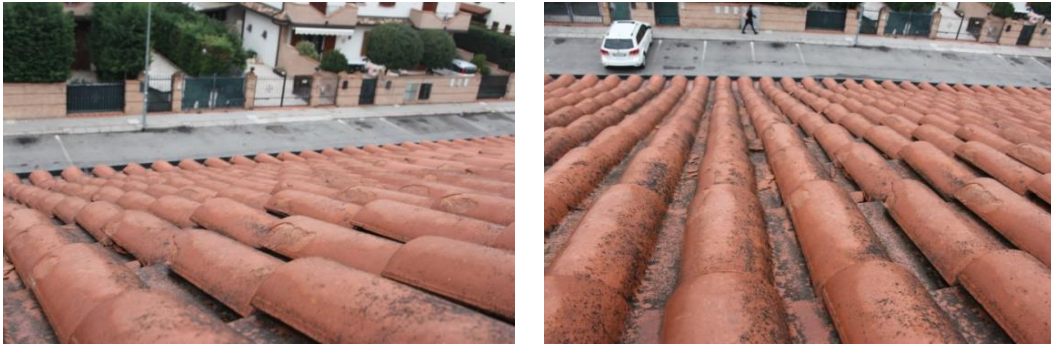
Figure 4.8 Deterioration of the shingles
