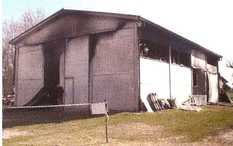
Figure 4.28 Partial collapse of a building due to a fire
