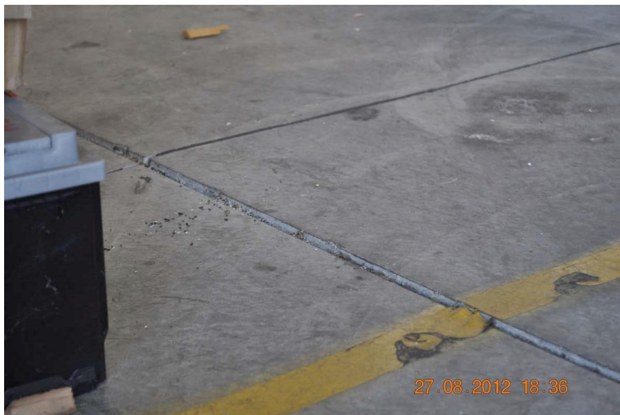
Figure 4.33 N° R.G. 10141/2012 Curling of a concrete slab
