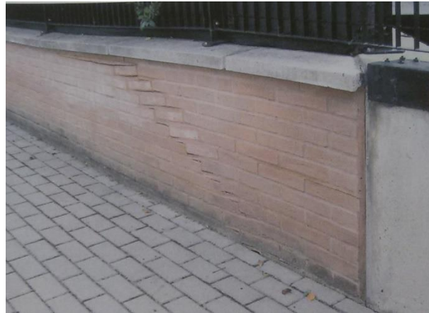
Figure 4.11 Cracks on a masonry enclosure
