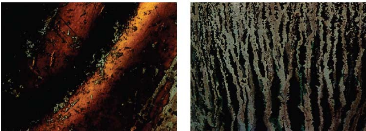
Fig. 22. Typical alternation of light and dark areas of surface corrosion[26]
