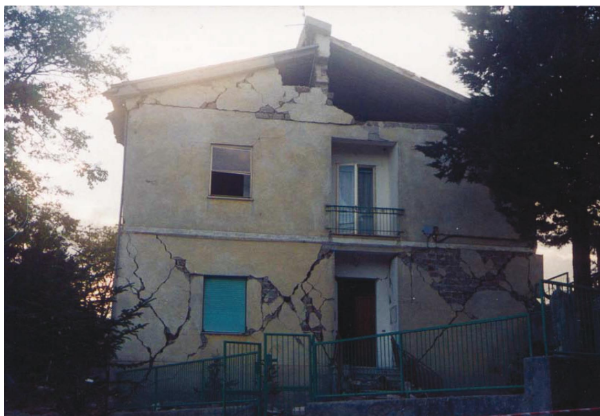
Figure 1.3: Example of “second damage mode” mechanism (from http://ww2.unime.it/ingegneria/new/materiale )
