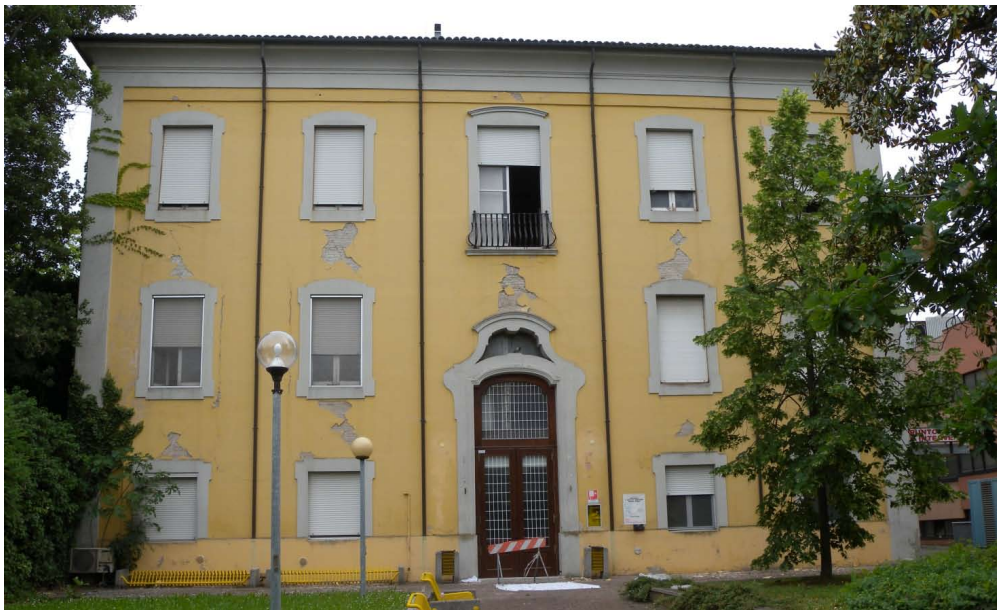
Figure 2: Finale Emilia hospital, after the earthquake that stroke Emilia-Romagna region (Italy) in May 2012. Wide cracks opened in the spandrels (from http://www.eqclearinghouse.org )
