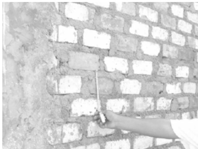
Figure 1 Thick of mortar bed joints
