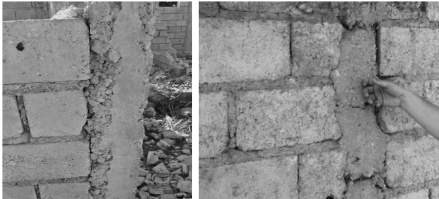
Figure 12 Unconsolidated concrete at the interface with masonry
