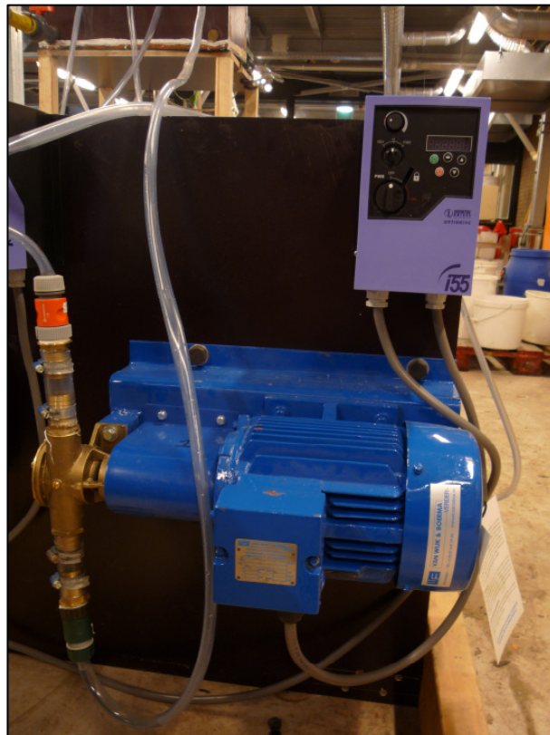
Figure 2.13 - Pump with a frequency regulator.
