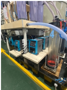
Figure 8: safety containers and pumps support
