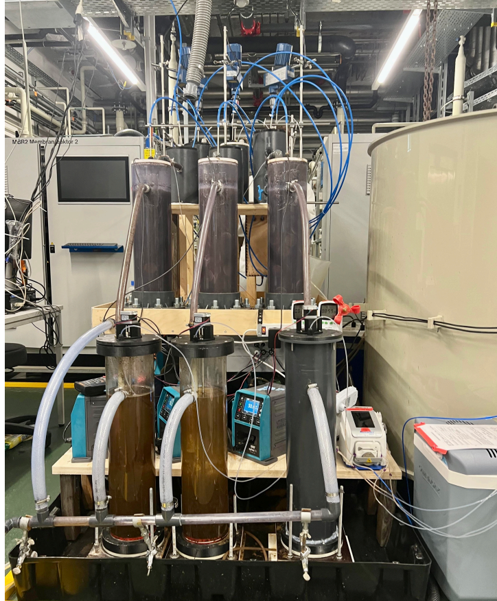
Figure 2.1.4: Overview of the pilot plant in the PTC during operations.
