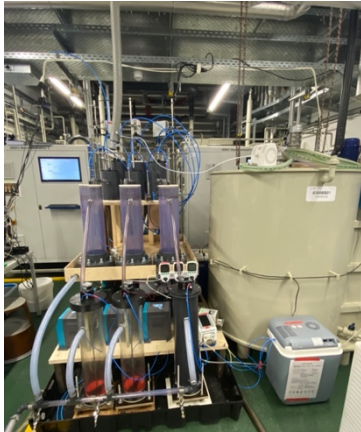
Figure 4: overview of the pilot plant
