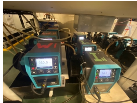
Figure 7: Watson Marlow Qdos60 pumps
