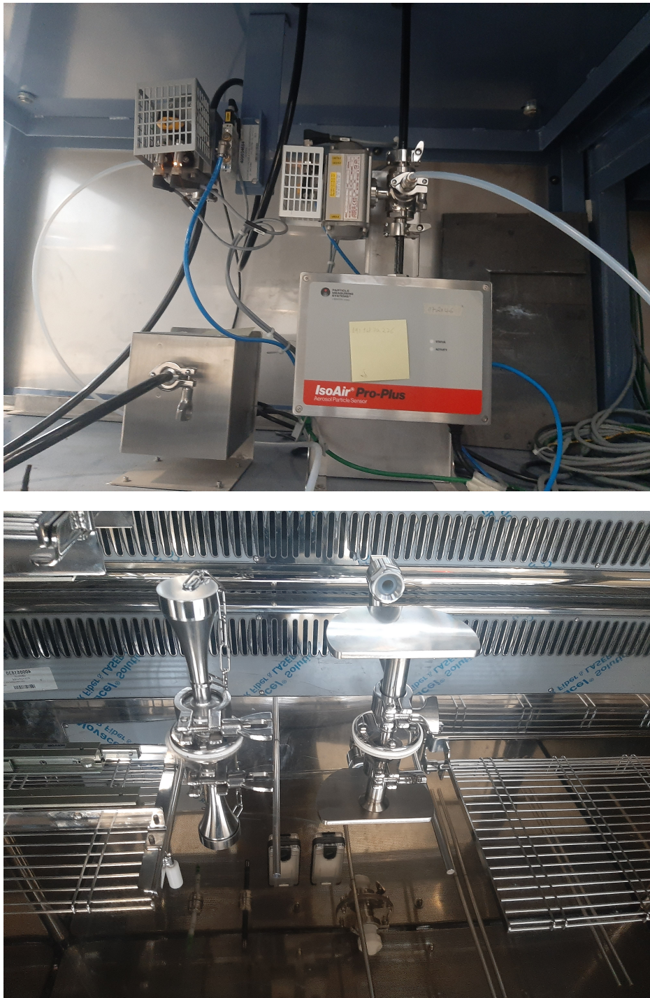
Figure 3.6: IsoAir Particle sample/Microbial installation.
