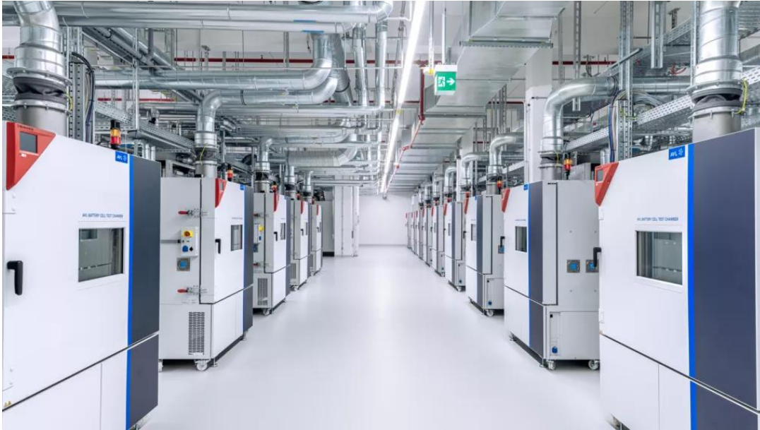
Figure 64 - AVL Battery Cell Test Chamber [29]
