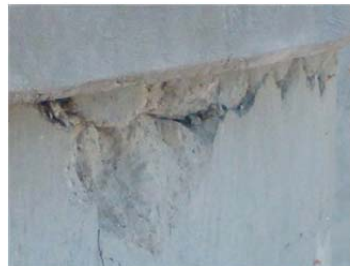
Fig. 1.1.10: Concrete spalling (a) at the roof-wall joint (b) at the base.
