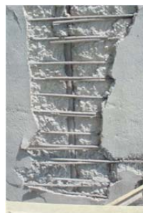
Fig. 1.1.11: (a) Silo with extensive spalling and exposed rebar (b) Close up of exposed rebar.
