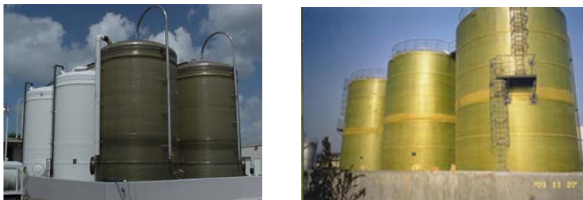
Fig. 3.1.2.6: Examples of tanks wrapped with FRP laminates.
