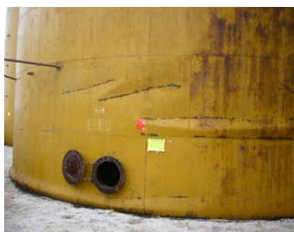
Fig. 3.1.2.1: “Elephant’s foot” buckling in a tank, Pisco earthquake, Peru, 2007.
