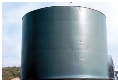
Fig. 3.1.2.2: “Elephant’s foot” caused by the movement of water in a large steel storage tank during San Fernando, California, earthquake (February 1971).
