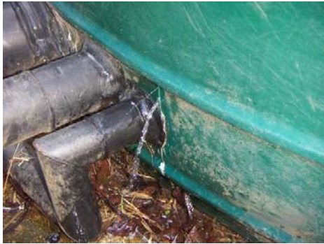
Fig. 1.1.7: Water loss due to breaking of tank-pipe connection.
