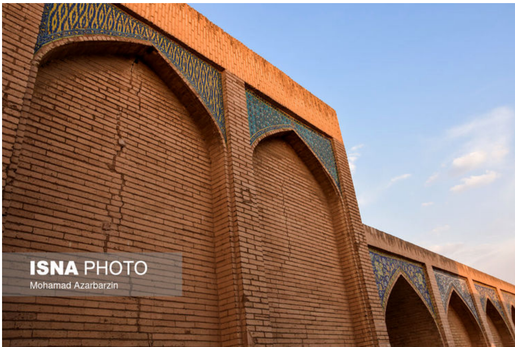
Figure 4-6: Cracks that are Recently Observed in Khaju Bridge (Source: ISNA)
