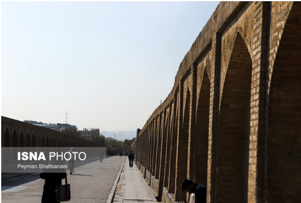
Figure 4-5: Damages Observed on Si-o-Se-Pol Bridge (Source: ISNA)
