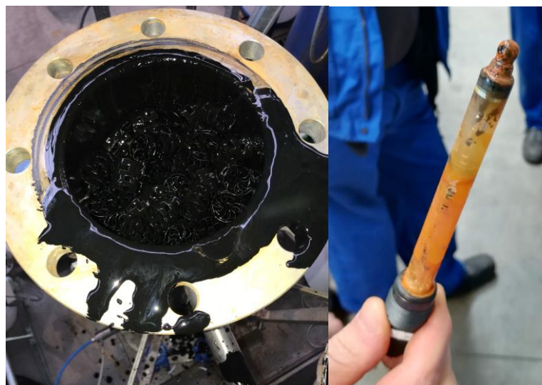
Figure 4.5: The accumulation of \text{FeS} in the scrubber column sticking all the rushing rings; the pH probe dirty and corroded by \text{Fe} solution.
