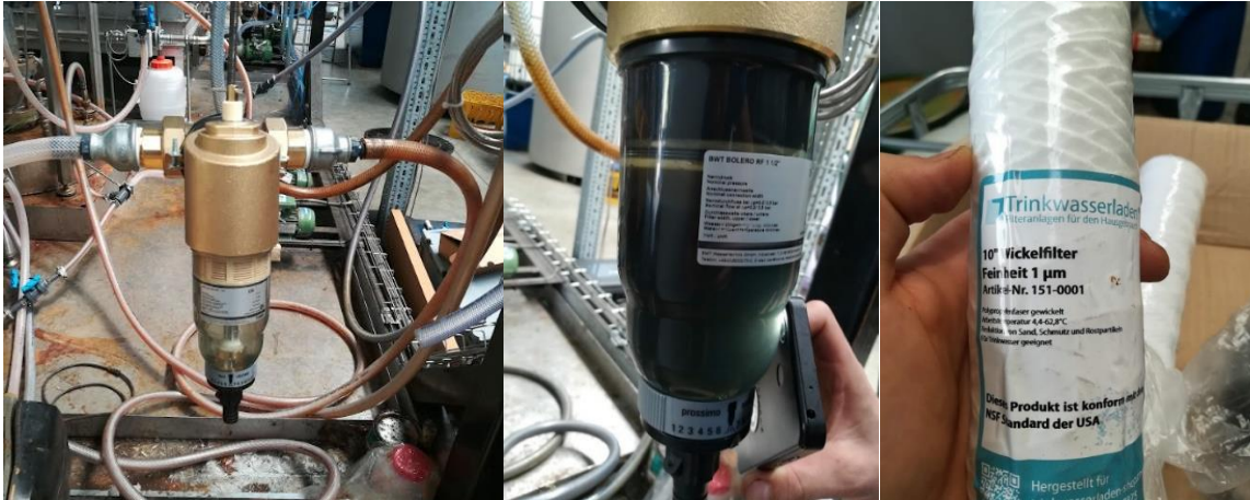
Figure 4.9: Before and after bolero filter workout; the new filter installed
