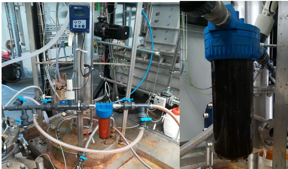
Figure 4.11 The new upgrades filter in the system: before and after the scrubbing activity the filter itself turns to black and dirty condition
