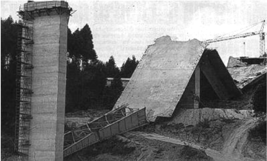
Figure 2.3: Injaka bridge collapse, July 1998, due to a poorly controlled construction process
