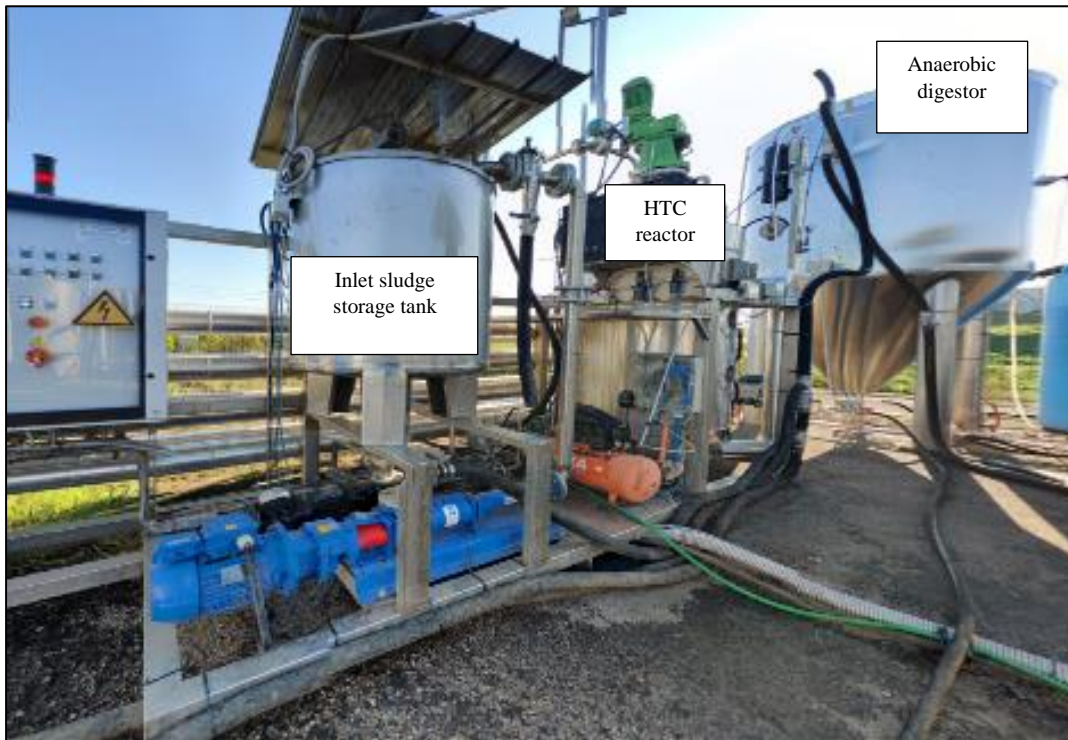
Figure 6: HTC unit and anaerobic digester.
