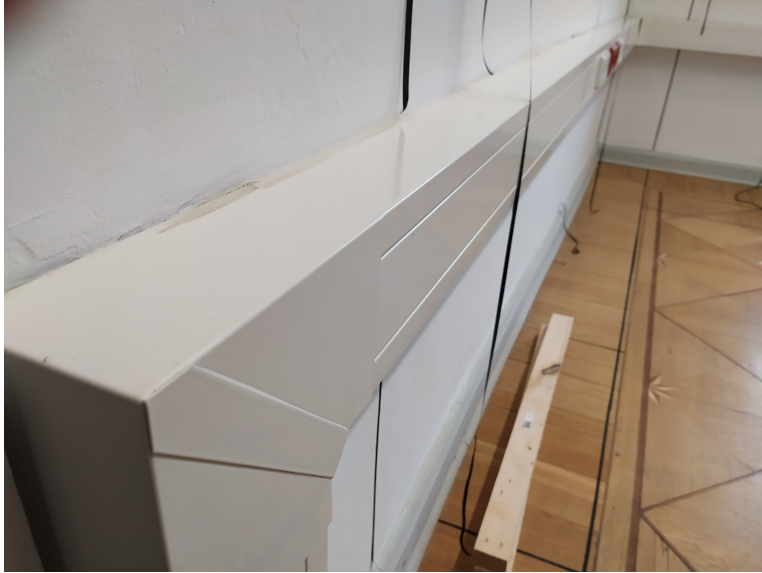
(a) Cable duct.
