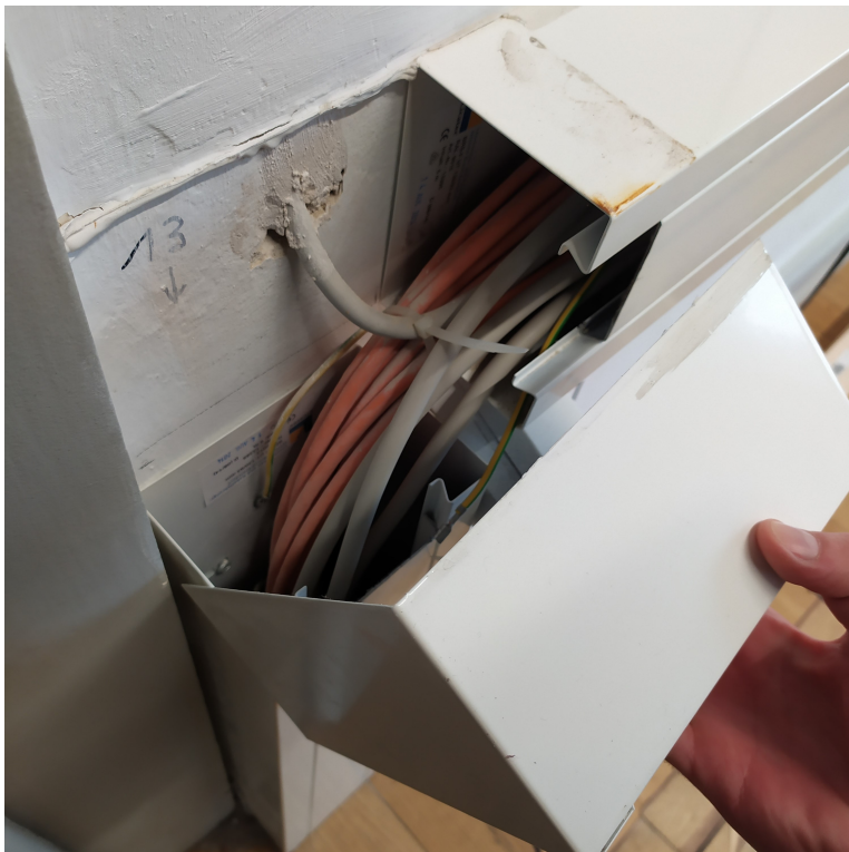
(b) Detail of the cables inside the duct.
