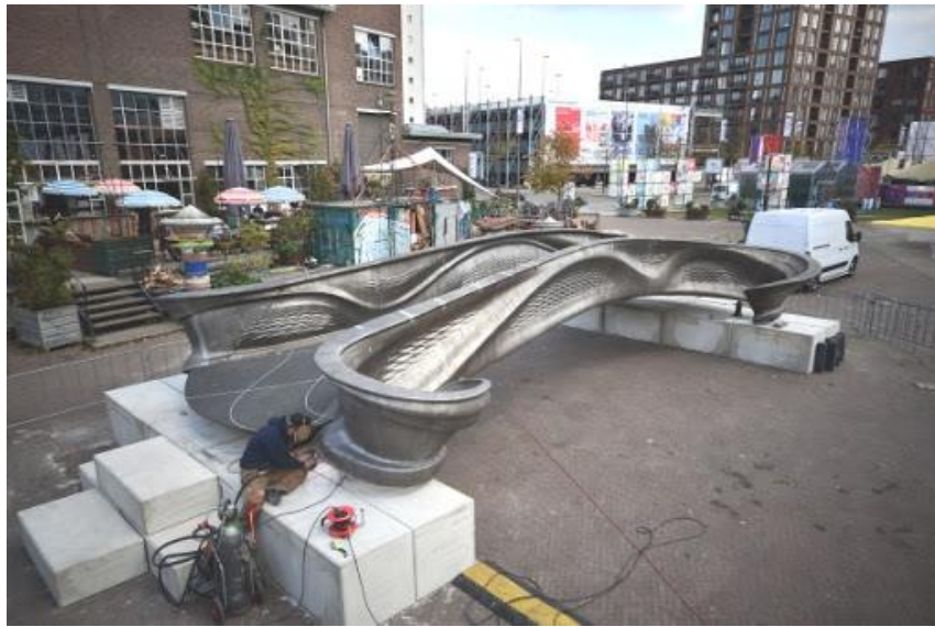
Figure 43: (a) The Frame (Top) and (b) The Completed Form (Bottom) of MX3D Bridge
