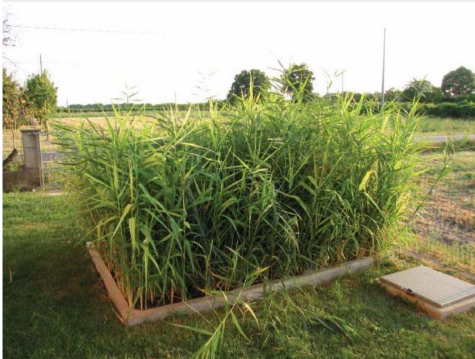
Figure 9: Constructed wetland for treatment of domestic wastewaters coming from isolated house (2 PE) (Lajo, s.d.)
