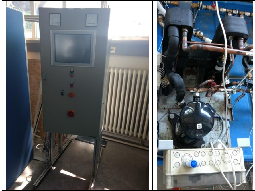
Fig. 61 - Electric panel (left) and heat pump (right)
