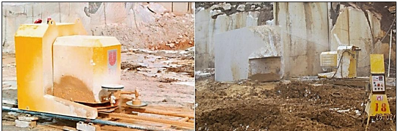
Figure 9 Dazzini Diamond Wire Marble Cutting Machine
