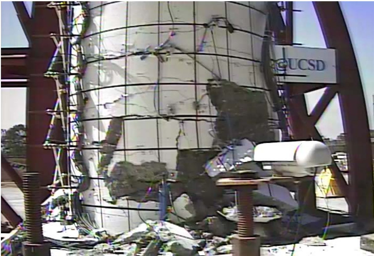
Figure 4.51: Column base post-EQ5
