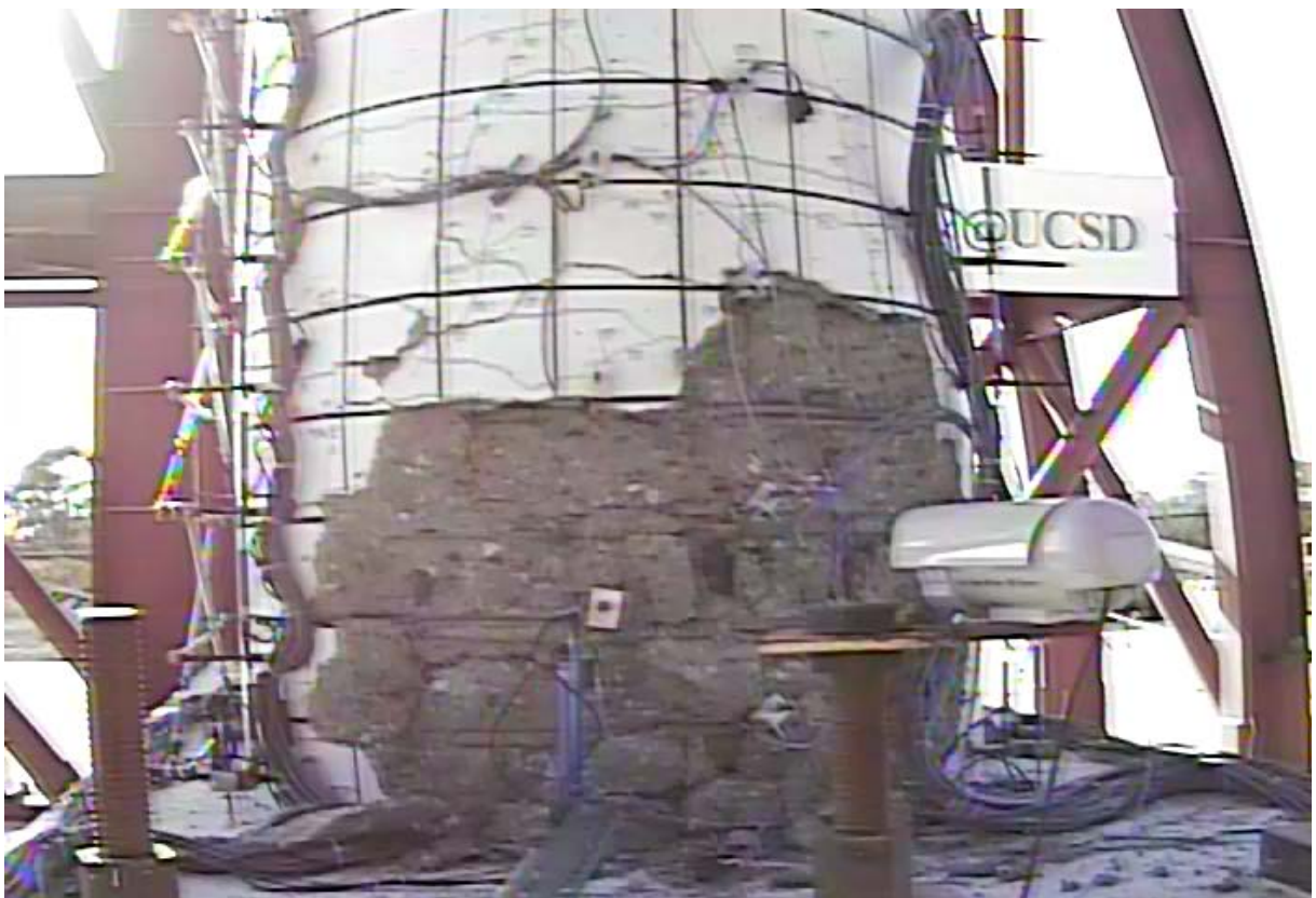
Figure 4.75: Column base post-EQ7
