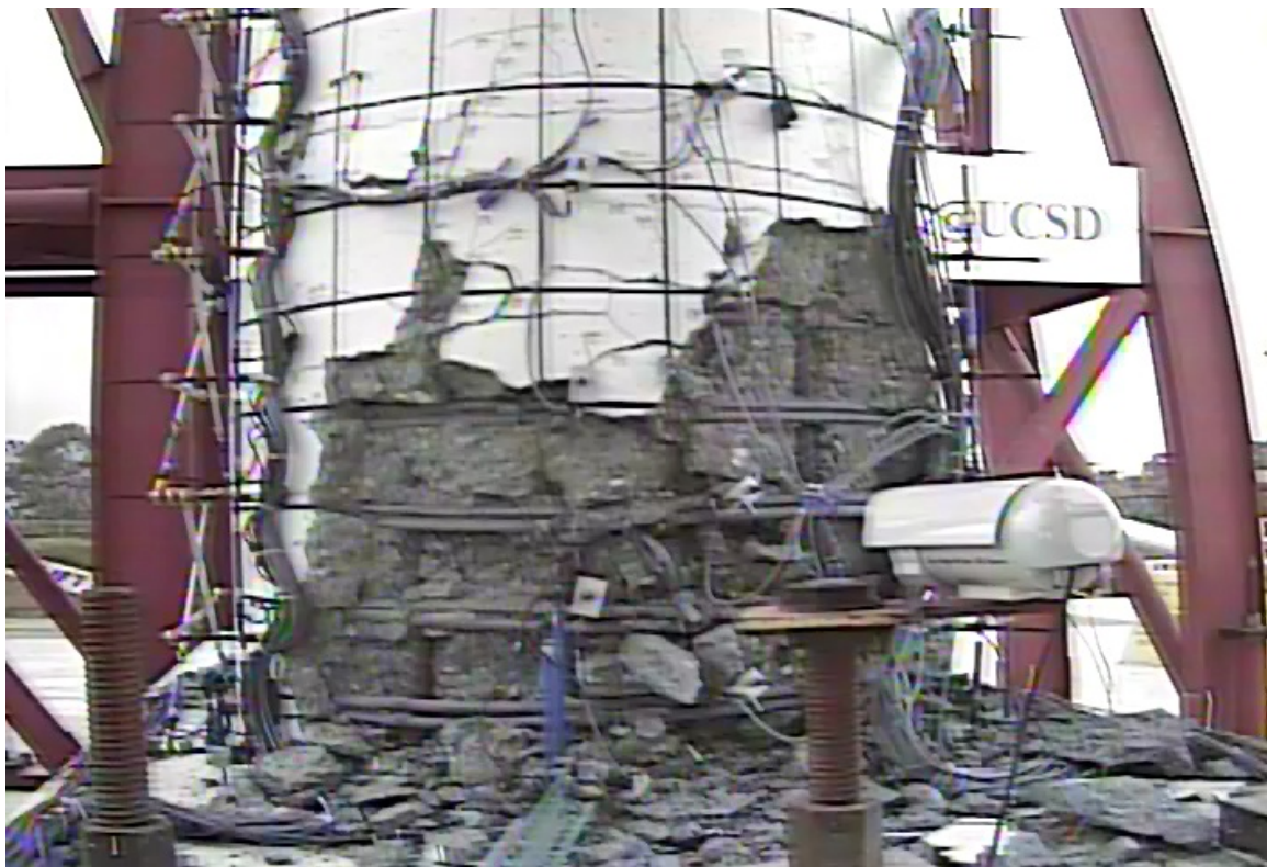
Figure 4.99: Column base post-EQ9
