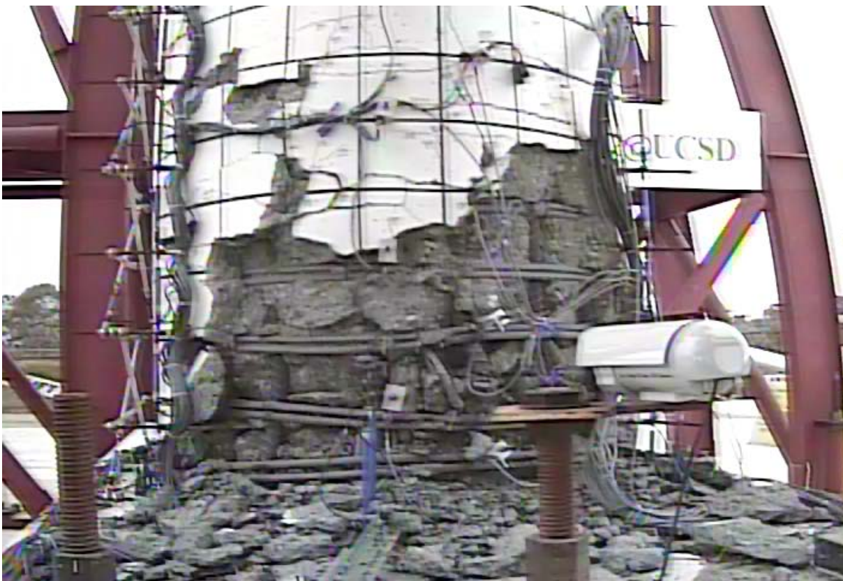
Figure 4.111: Column base post-EQ10
