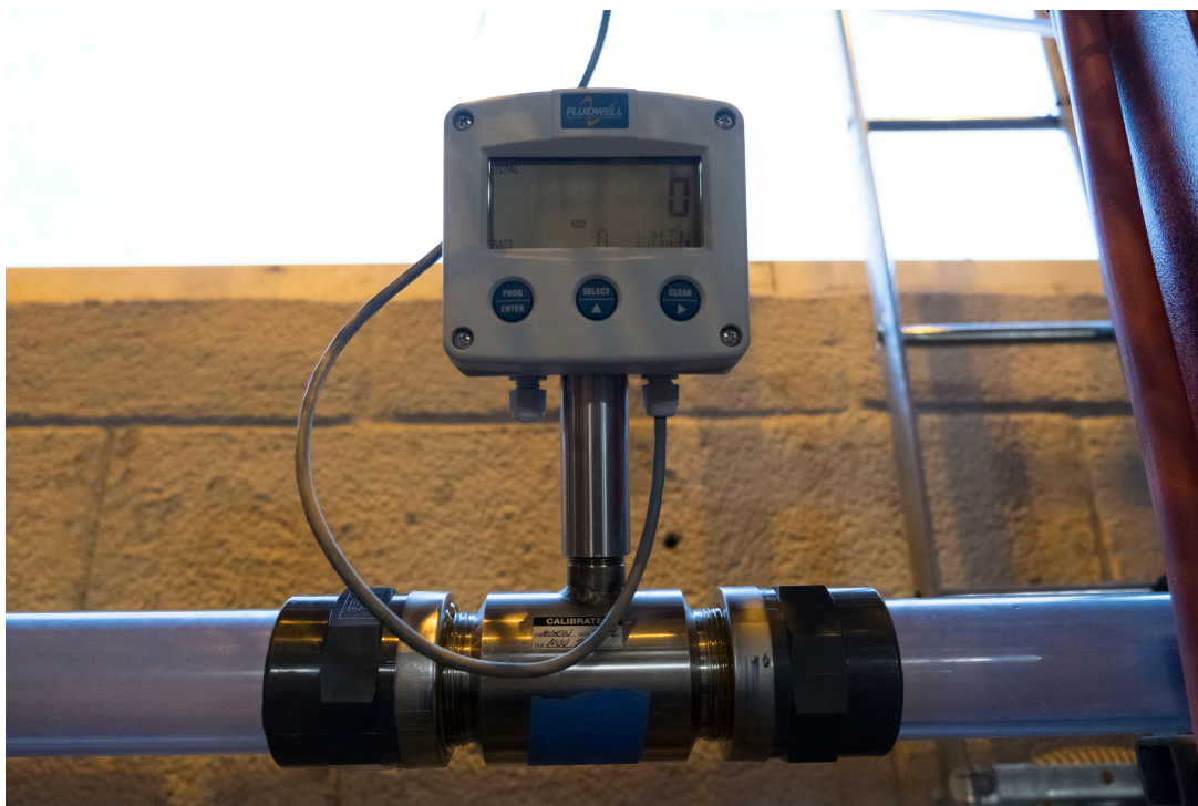
Figure 4.14: Flow meter installed on the flushing rig.
