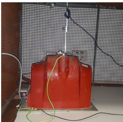
Fig 3.11: The step-up voltage transformer. At left there is the low voltage primary side while on the top there is the secondary high voltage bar.
