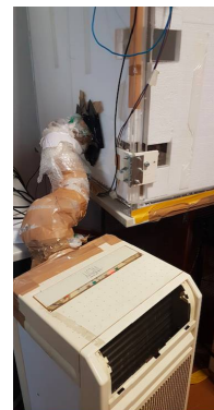
Fig. 3.17: The portable air conditioner connected to the thermostatic chamber.
