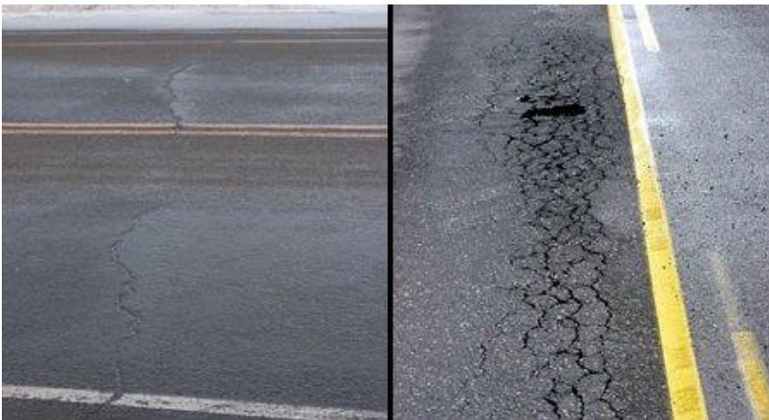
Figure 1.12 -Loss of aggregate
