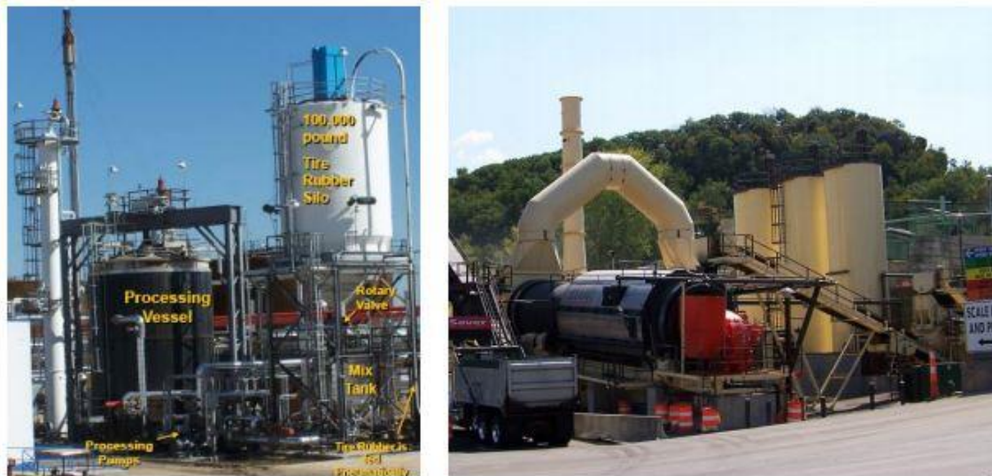
Figure 2.14 -Terminal Blend CR (left); Mixture production plant with vertical binder storage tanks which allow for better agitation and storage (right).
