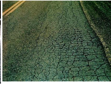
Figure 4.11 -Very severely fatigued cracked pavement
