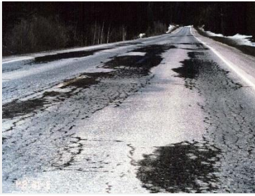
Figure 4.10 - Fatigue cracking as a result of frost action
