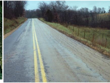
Figure 4.12 -Fatigue cracking from a lack of edge support
