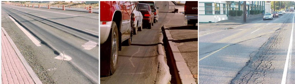
Figure 4.1 -Severe mix rutting.
