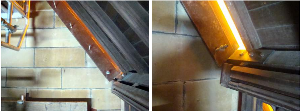
Figures 4.21, 4.22. Steel plates 200x12 mm welded at the end and M20 bolts, used to connect the front and back gables to the roof structure at the purlins
