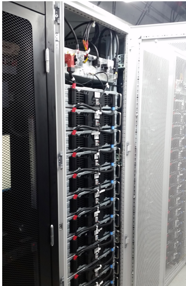
Fig. 4.3: Detail of two rows of batteries (courtesy of Entergy Inc.)
