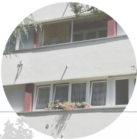
PERMANENTLY ENCLOSED BALCONIES
