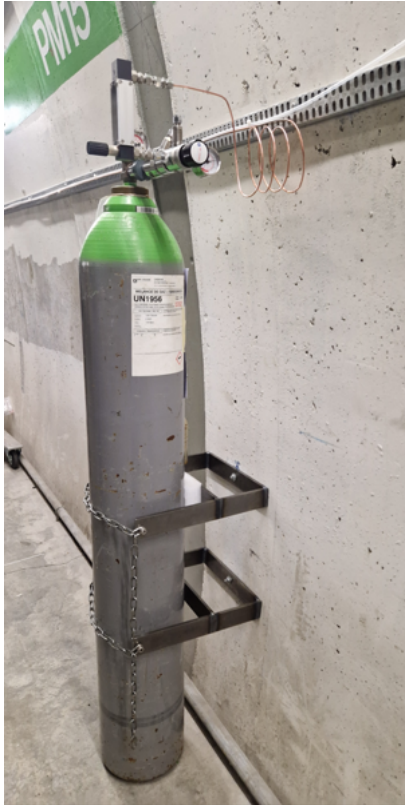
Figure 3.14: The gas bottle for the MiniDT gas circuit, fixed to the UJ18 wall. The copper tube transports the gas mixture to the MiniDT Y, while the plastic tube is the return flux, that ends in the gas bubbler.
