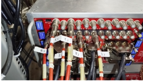
Figure A.2: The MiniDT power booster, with the CAEN A7030DN module for the cathodes ( -1200 V) and a CAEN A1833P for the strips and anodes ( +1800 V, +3600 V respectively) and the corresponding HV cables.
