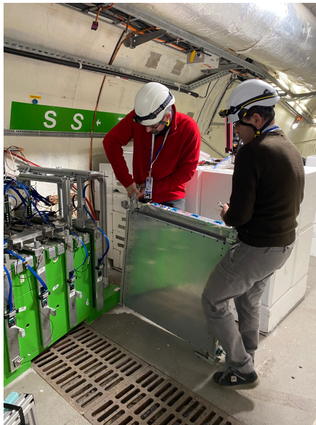
Figure 3.9: Placement of MiniDTs in the mechanical support structure.
