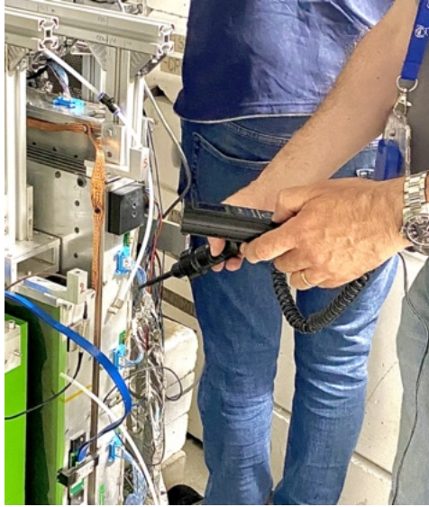
Figure 4.19: The CO 2 detector, used to find the gas leak on MiniDT Y. The black box, visible next to the detector, is the MiniDT Y LVFE box, the one that caused the leak in the MiniDTs system.
