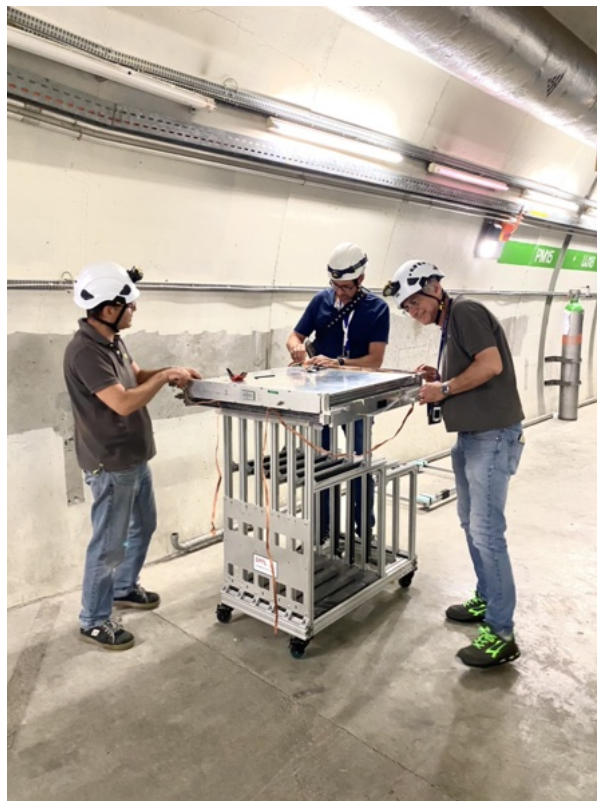
Figure 4.20: The extracted MiniDTs before the MiniDT Y substitution, being stripped of the grounding braids and slow control services, to move them to the spare chamber.
