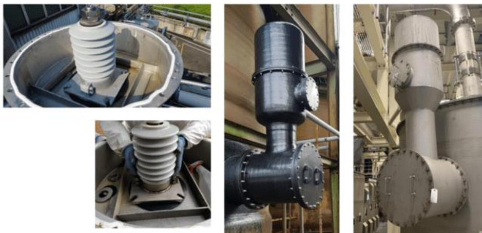
Figure 7: insulating sectors and ceramic insulators
