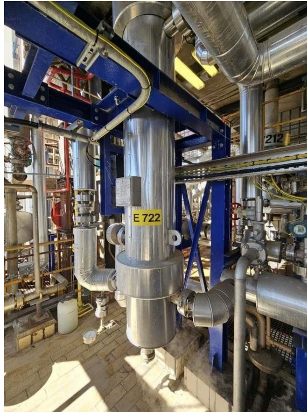
Figure 34: heat exchanger E722
