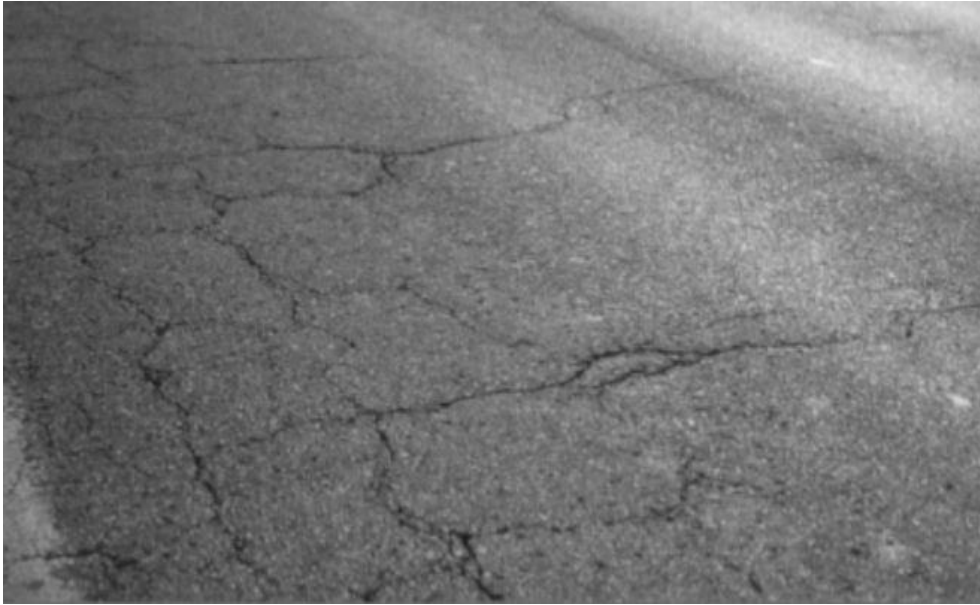
Figure 2.3: Longitudinal Cracking (Medium Severity)
