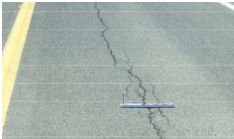
Figure 2.6: Longitudinal Cracking (Medium Severity)
