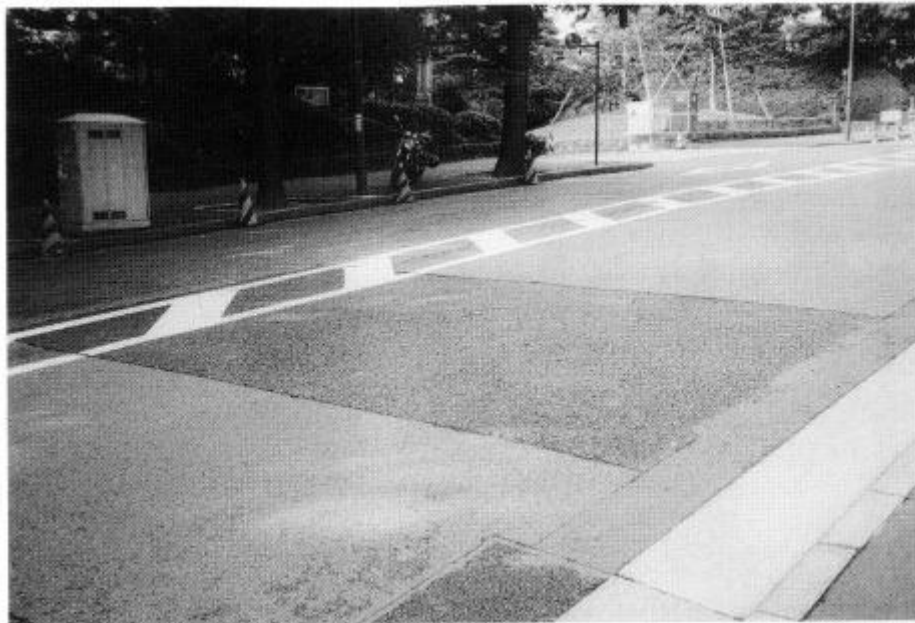
Figure 4.2: Pavement Distress Patch
