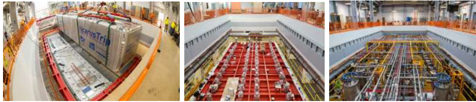
Figure 3.4: (Left) Deployment of the ICARUS cryostats in the pit of the SBN Far Detector experimental hall at Fermilab occurred in August 2018. (Center) The installation of TPC, PMT, and laser feed-through flanges followed in December 2018. (Right) The ICARUS detector was ready at the start of data taking for commissioning.
