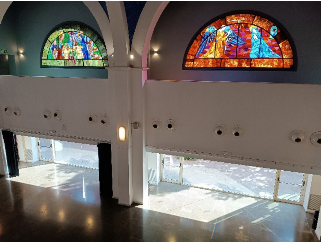
Figure 37. Above: Audience area, seats located within the central part of the hall Below: curtains left opened due to a malfunction.
