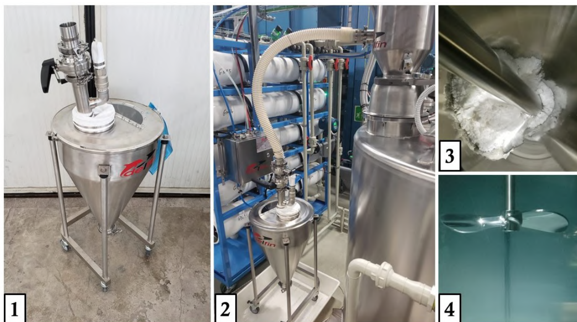
Figure 4.6: Pictures of all the elements needed for the insertion of Gadolinium salt inside the GdWPS: hopper for the Gd transport (1), connection to the pneumatic system above the mixing tank (2), lance which helps catching the salt inside the hopper (3) and stirrer inside the mixing tank which mixes the solution (4).
