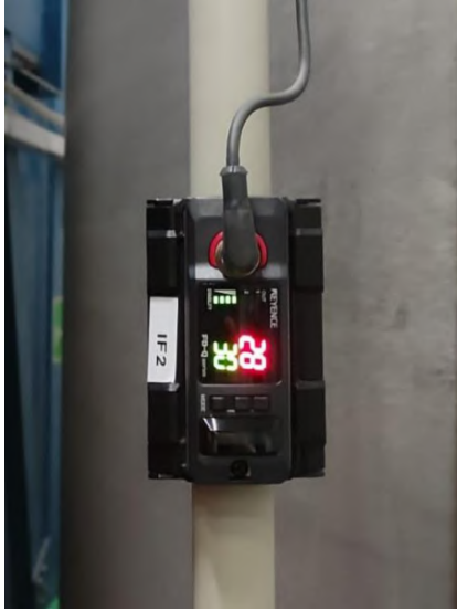
Figure 4.11: Picture of one of the ultrasonic flow meters (IF2) used in the GdWPS.
