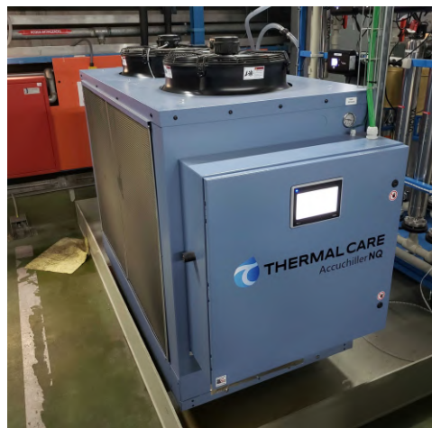
Figure 4.5: Picture of the GdWPS chiller. In front of it, the control display acts as interface to the user; on the top, the two fans are used as vent.
