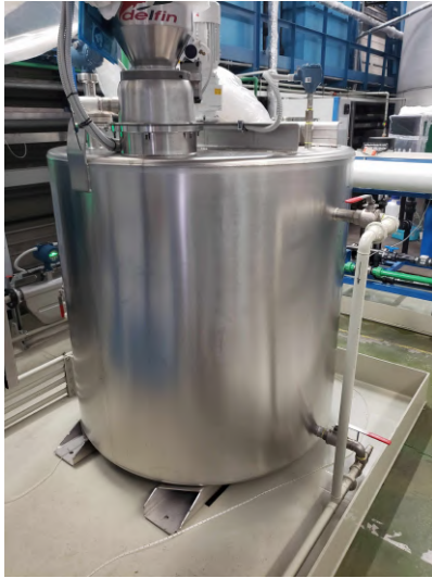
Figure 4.3: Mixing tank of the GdWPS. The Gd sulfate is inserted by the top (see next Section). It holds 2 tons of water and has four input lines and two output lines (on the right in the picture).
