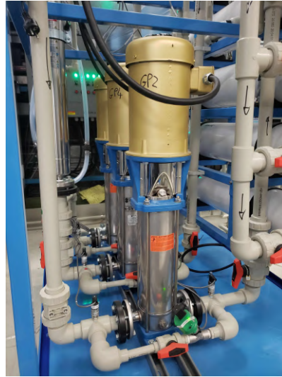
Figure 4.4: One of the pumps of the GdWPS. In front of it, the corresponding bypass line with the solenoid valve adjusting the pump intensity.
