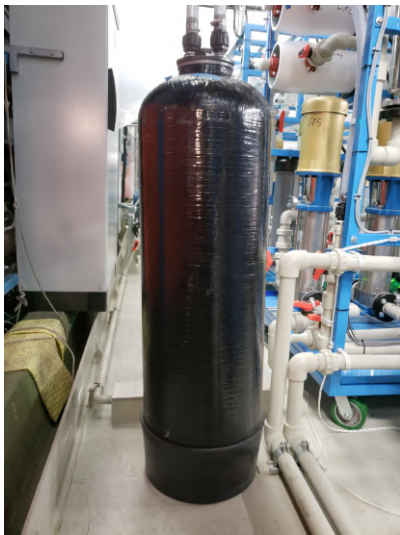
Figure 4.9: Picture of the black tank holding the resins used in the GdWPS. The two flexible tubes on the top are the input and output lines connected to the plant.
