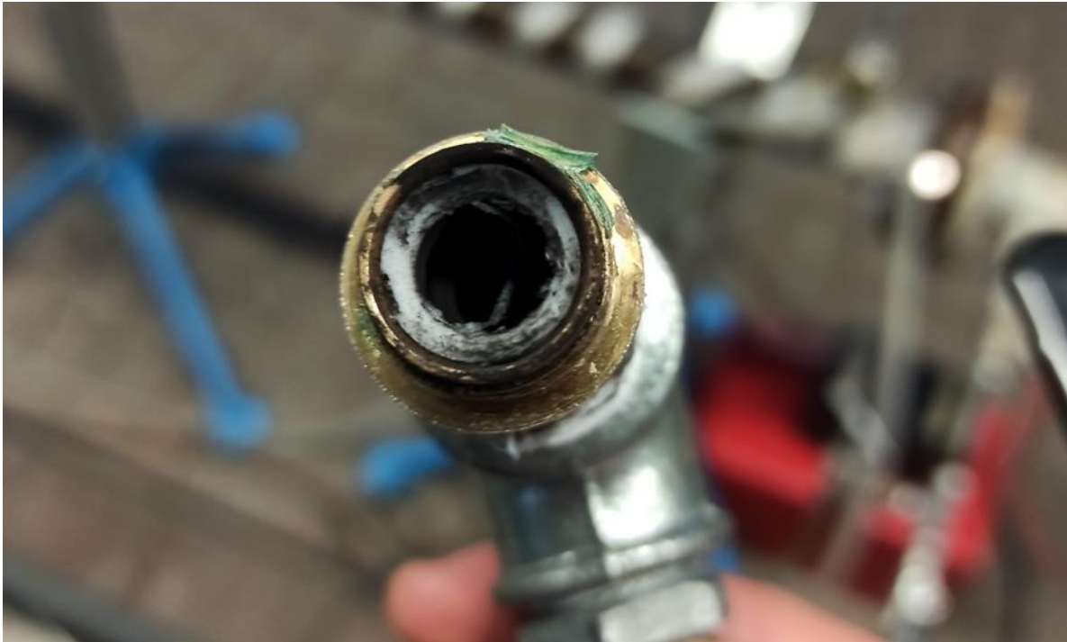
Figure 32 - Damaged valve seal
