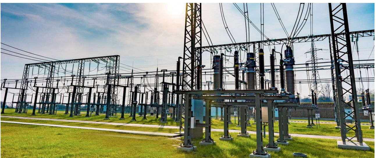
Figure 1: EHV Substation – FIATO Substation
