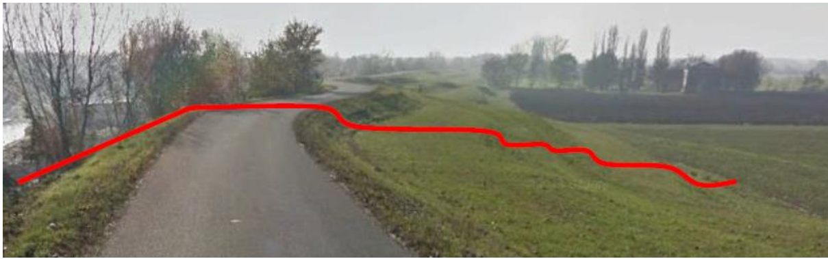
Figure 44: Images taken from Google Earth, example of berms series of a levee
